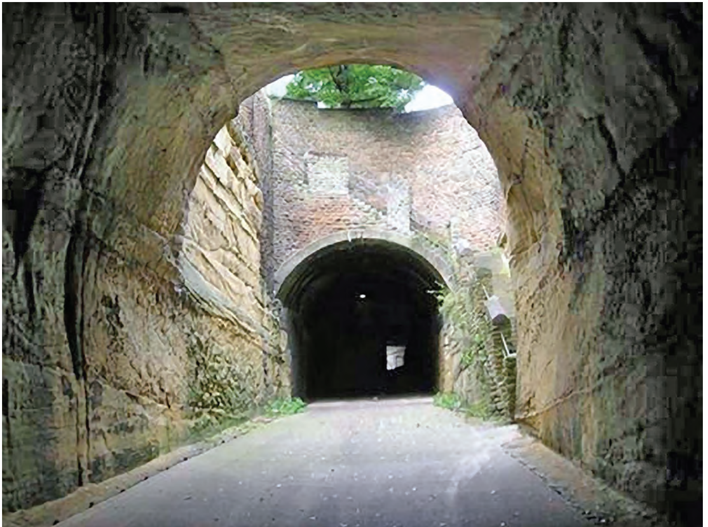
The Park Tunnel in Nottingham showing the light well and steps up to street level
